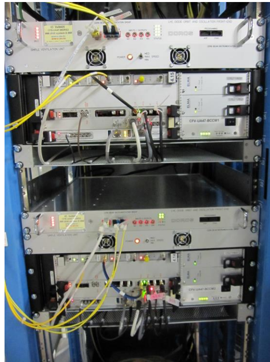
Fig. 1: A photograph of BCCM electronics accommodated in rack BY05 in UA47. From top to bottom: BCCM front-end A, a ventilation unit, VME crate A, BCCM front-end B, a ventilation unit, VME crate B. Two CIBU modules for systems A and B are not visible in the photograph and are located at the bottom of the rack.
