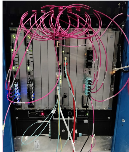
Figure 9: Hardware demonstrator of the track finding output running on the board on the left outputting tracks over five fibre optic links to the vertex finding running on the board on the right where the vertex is calculated and stored in buffers.
