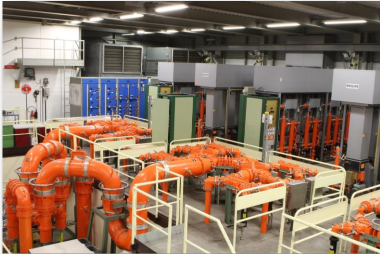
3 dB combiner 32 x 35 kW to 1 x 1 MW (~ 50 m 2 )
