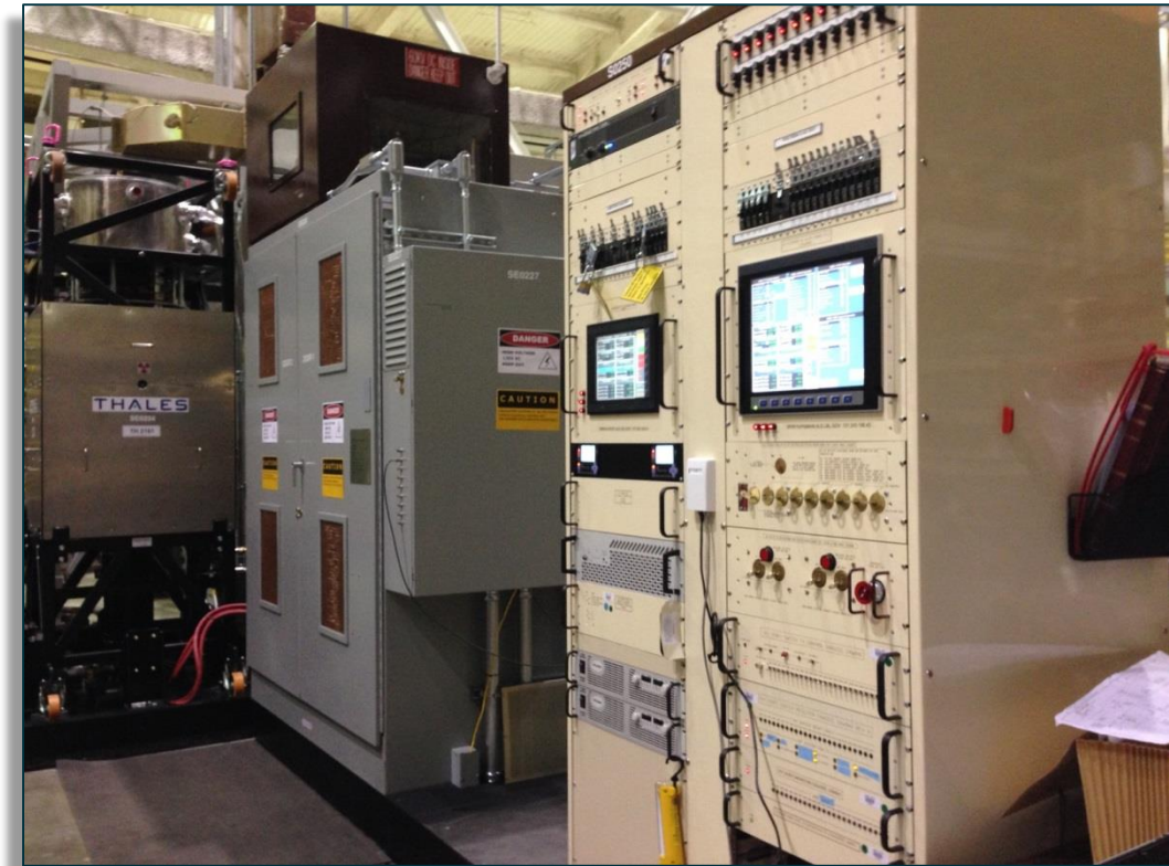
Filter Cabinet and PLC Controls
