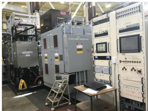
Klystron site 1 with -56 kV HV switch
