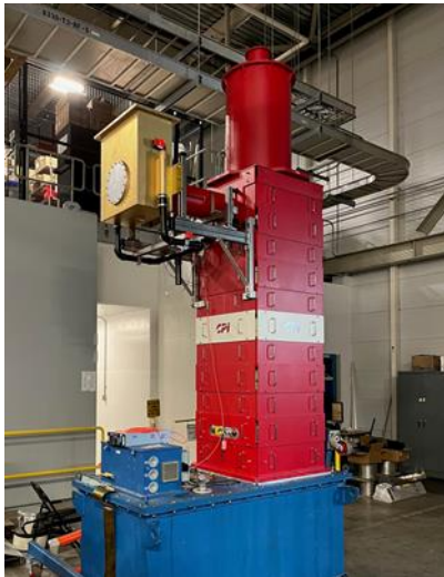
New 3 MW klystron first article in SNS Radiofrequency Test Facility (RFTF)
