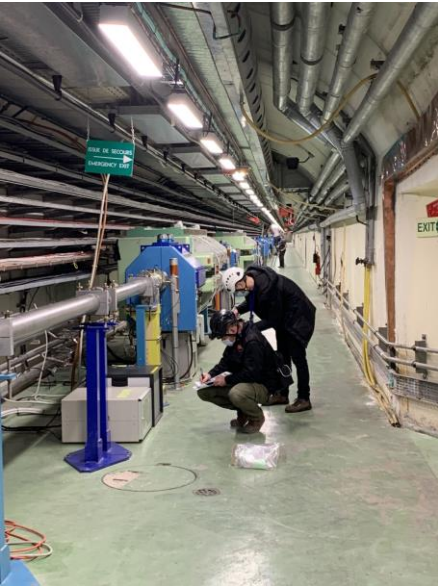
RPL installation in transfer lines
