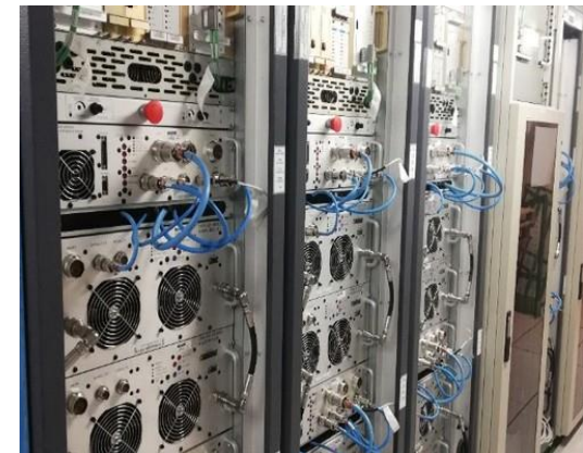
Converters installed in LHC (104x)
