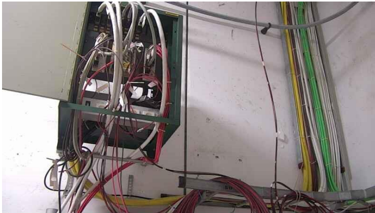
North Area BLM cables connection In place 50 minutes after the call
