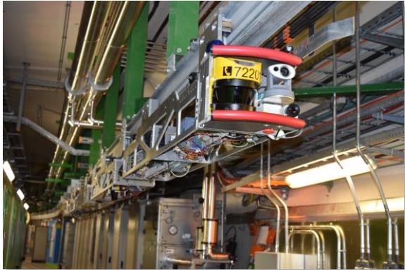
Train Inspection Monorail [10] (CERN made)
