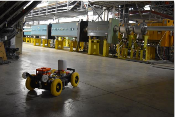
EXTRM robot (CERN controls)
