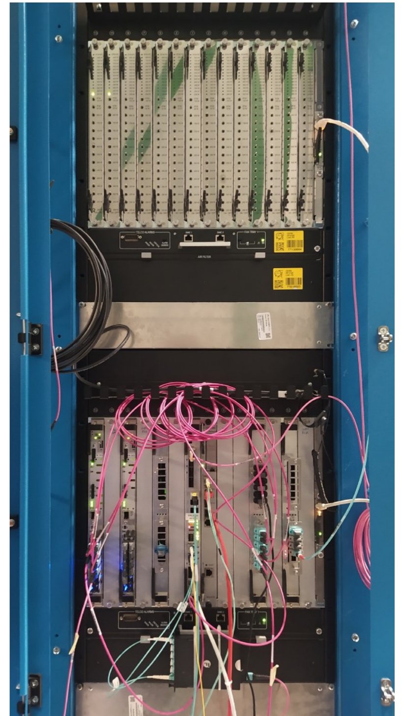
Rack A16 in building 186 (Couple of months ago)
