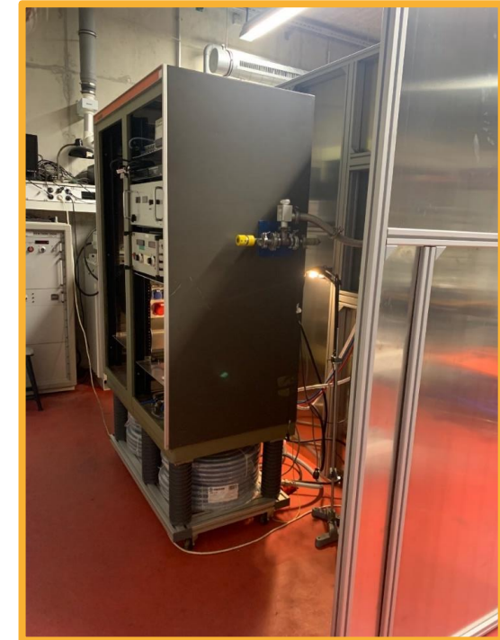
HV terminal inside cage
