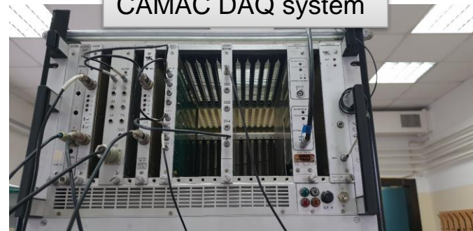
CAMAC DAQ system
