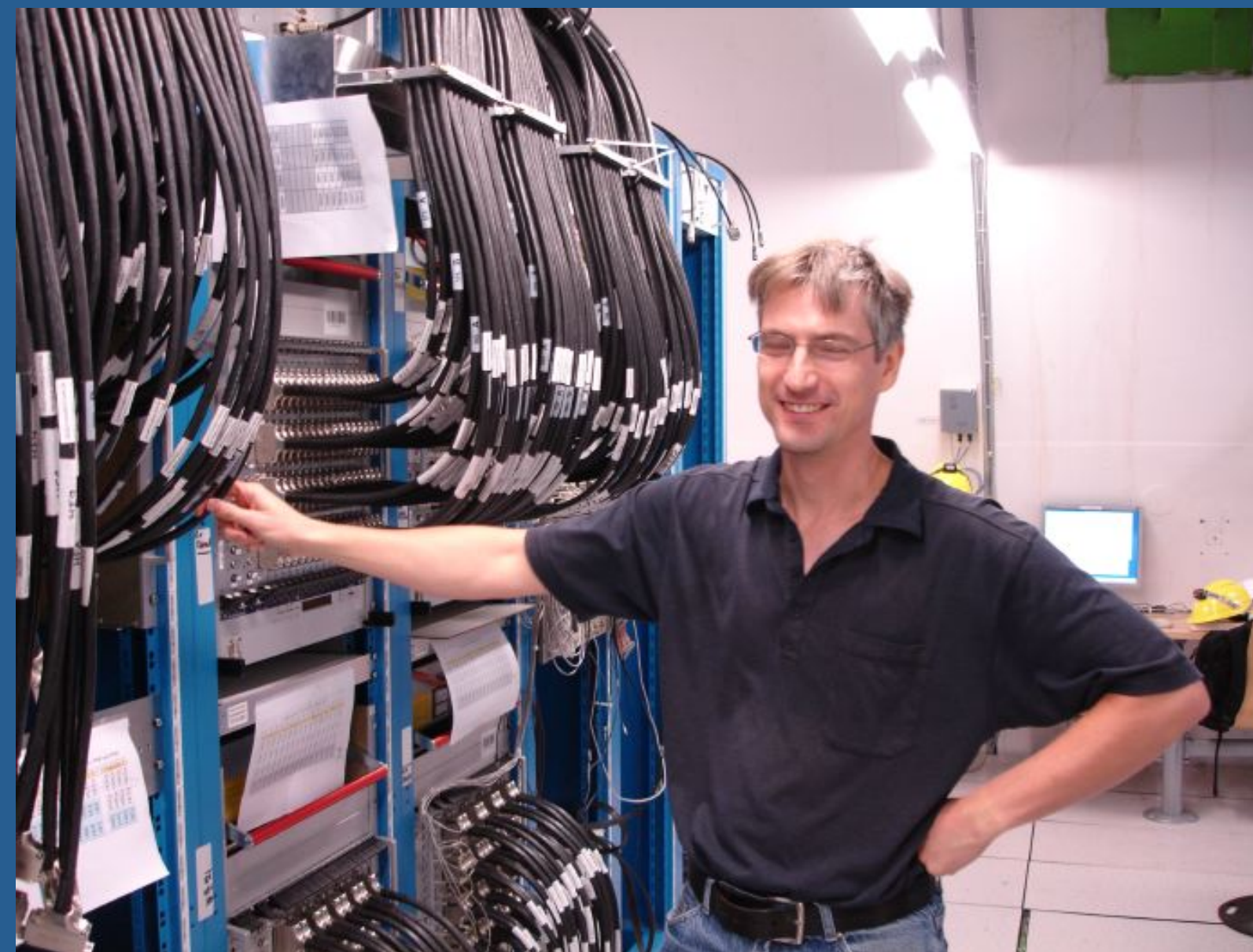
Steve with a lot of cables
