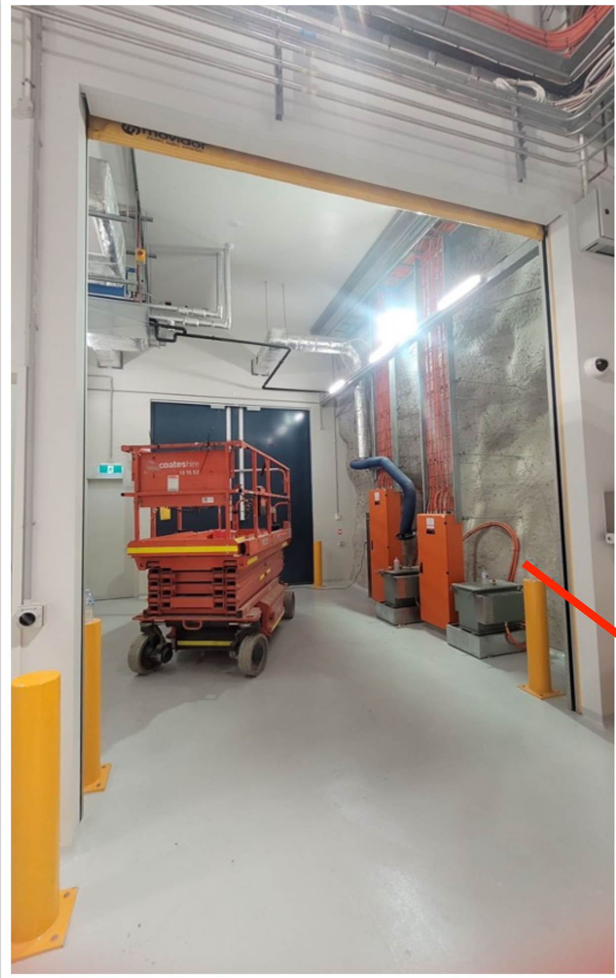
Ante-Room for equipment Clear
