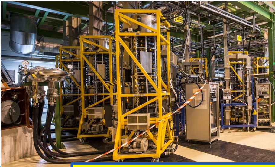
The LHC cavern UX45 with the klystron gallery.
