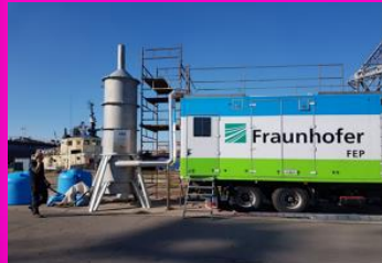
EBFGT installation at Riga Shipyard. Mobile accelerator (R) & wet scrubber (L)
