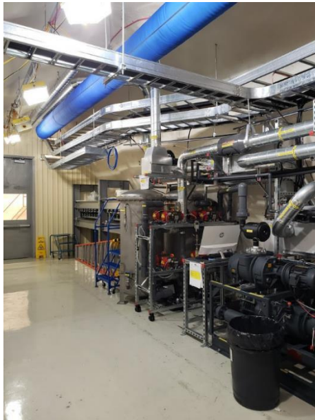
Radon filter system
