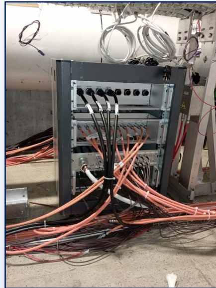
Proposed Rack to be installed
