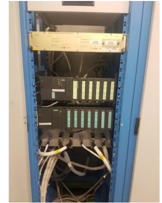
PLC for temperatures monitoring
