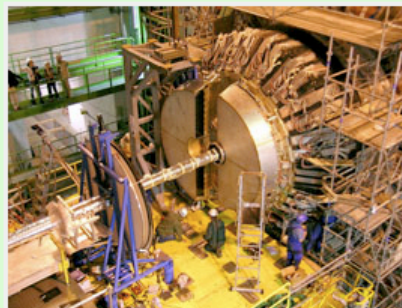
Approaching Dee2 to Dee1 with a very small clearance was one of the most difficult operations in the mechanical installation. Copyright: STFC
