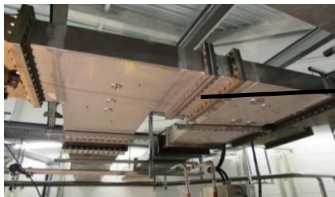
Waveguide network layout to power one or the other CM with 300 kW / cav from the 4 SSPA's, combined by pairs
