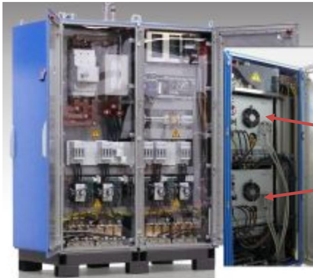
4x MOD-75 charger units = 300 kW
