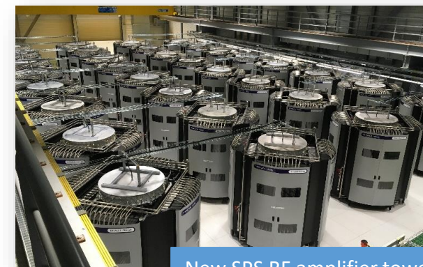
New SPS RF amplifier towers
