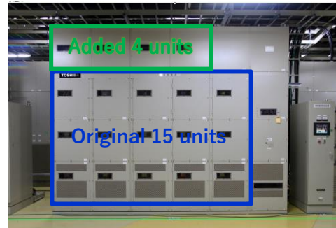
RCS RF Anode power supply
