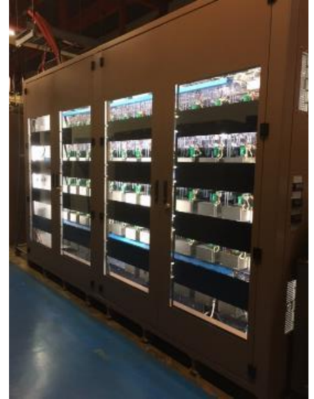
Marx Modulator Cabinet
