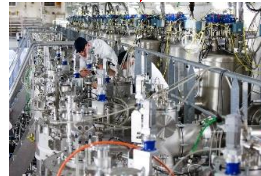
Cryogenic distribution system
