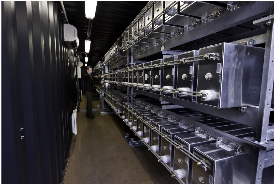
Capacitor banks for the 60 MW CERN-POPS power converter
