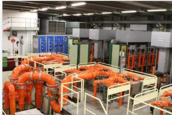
3 dB combiner 32 x 35 kW to 1 x 1 MW ( \sim 50 \text{ m}^2 )
