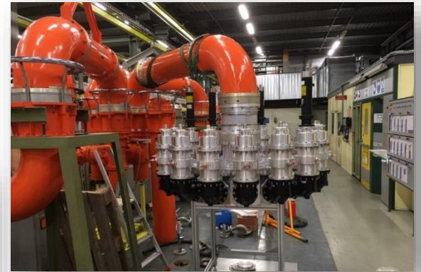
VHPCC (Very High Power Cavity Combiner) 16 x 70 kW to 1 x 1 MW ( \sim 3 \text{ m}^2 )
