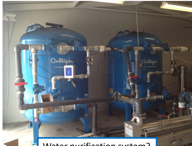
Water purification system?
