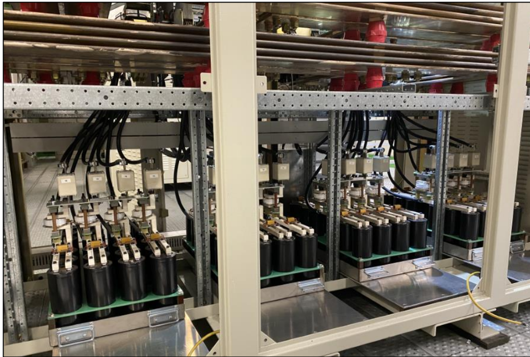
Snubber installed in CT-2 breaker
