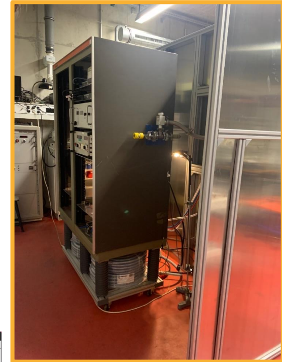
HV terminal inside cage
