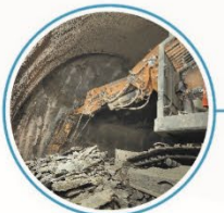
CIVIL ENGINEERING 2 new caverns, 1km underground galleries, two new large shafts; 10 new technical buildings on surface in P1 and P5 (near ATLAS and CMS)
