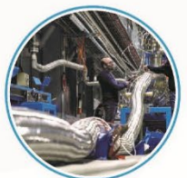
SUPERCONDUCTING LINKS 8 novel electric current superconducting lines, 140 m long and rated for 30-100 kA, based on M 0 B 2 superconductor operating at a temperature up to 20 K.
