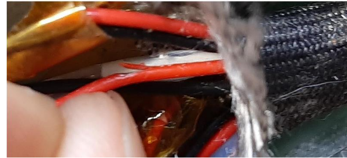
wire insulation damage at the end plate
