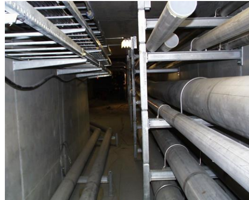
Industrial stainless steel piping
