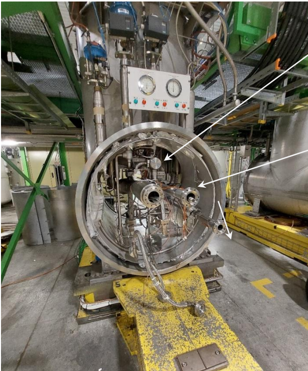
4x 2 kA Current Leads installed, individually tested
