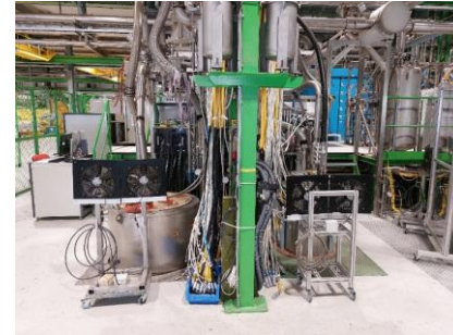
Proximity between Siegtal and diode
