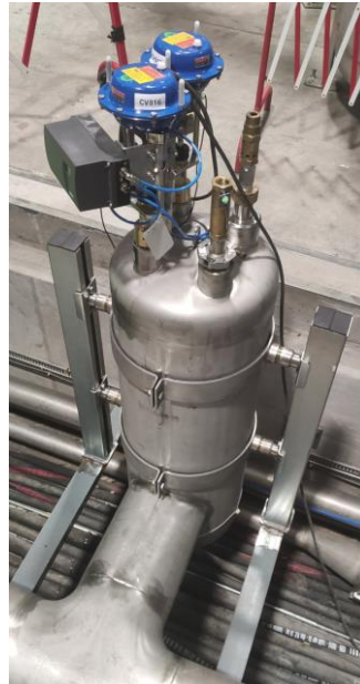
SVB Connected to SM18 Infrastructure
