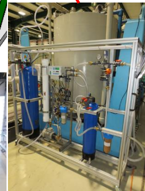
Cleaning facility by circulation
