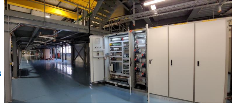
All electrical cryo cabinets installed in SM18
