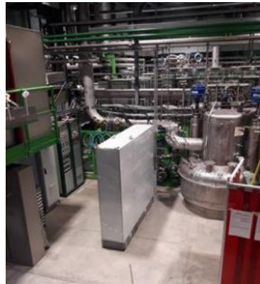
A. P. PCDS, CCU and heater unit cabinet
