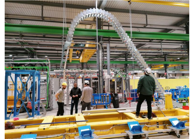
Existing cable chain at F2
