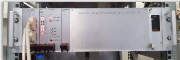
High level control unit
