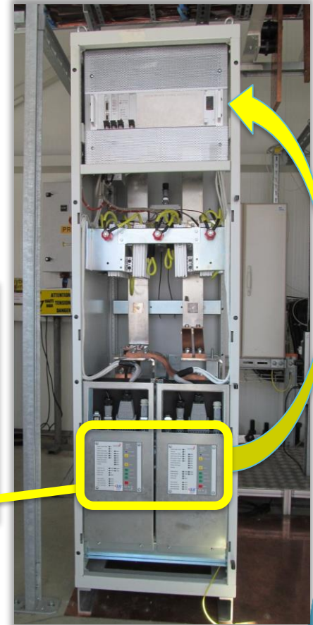
Local switch control unit
