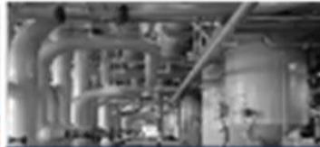
Complex piping For NI, TI & BOP
