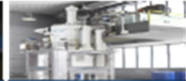
Waste Treatment equipment & facilities
