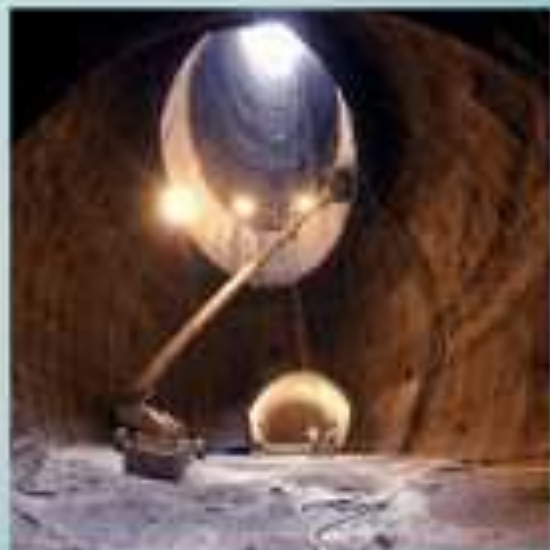
Shaft to the SSC tunnel at SSC, located at about 10 meters underground. The planned tunnel had a circumference of 87 km.
