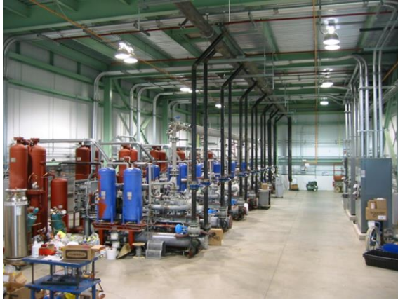
Figure 2. CMTF Warm Compressor building
