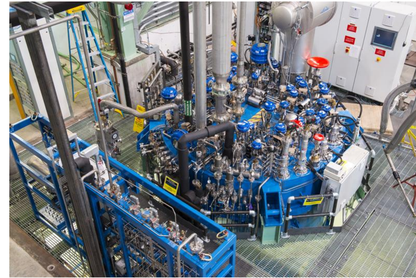
Superfluid Cryogenic Plant
