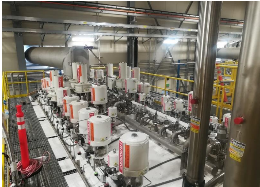
Cryogenic Valves on Lower 4K Cold Box
