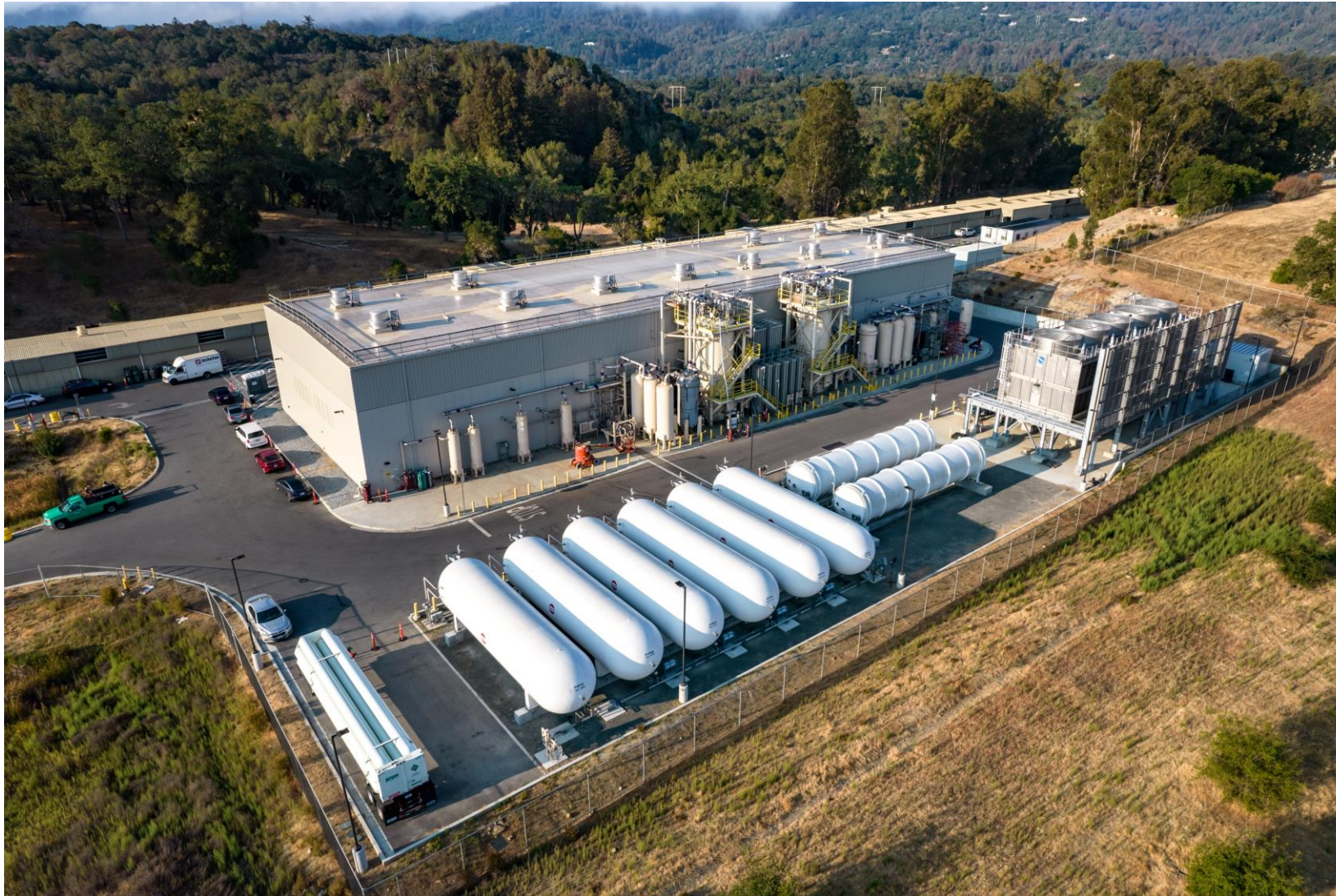
CRYOPLANT VIEW: GHe & LN2 Storages, Cooling Water and Vertical Cold Boxes.
