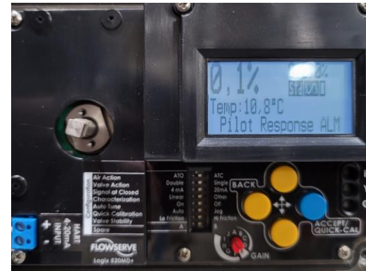
Failed CRYO Valve Positioner
