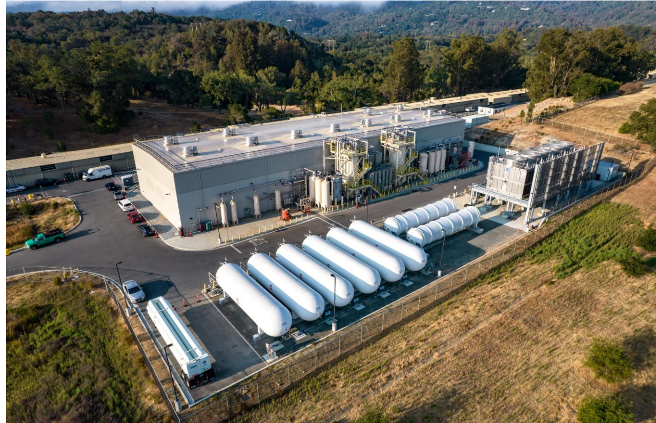
2023 - End of Commissioning
