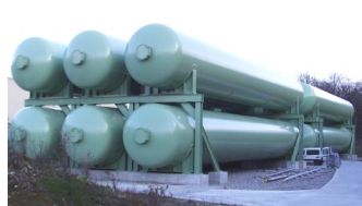
Liquid and gas helium storage
