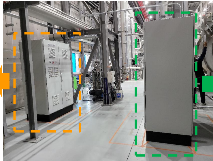
Vacuum pumping system panel (Electricity panel)
