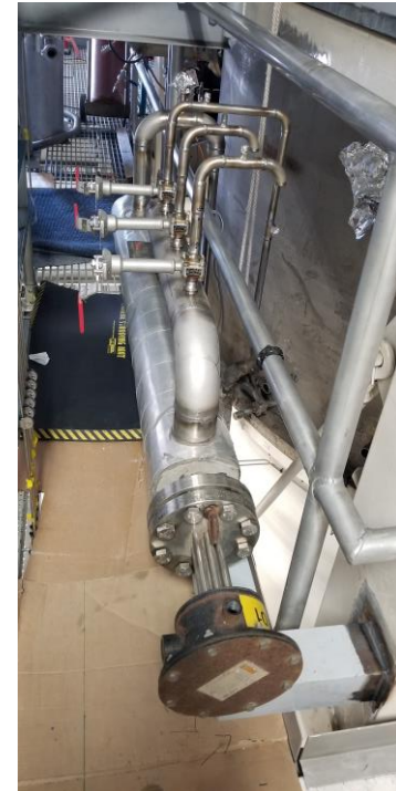
ESR2 Regeneration System for the 80 K and 20 K adsorbers at 4.5K cold box.
