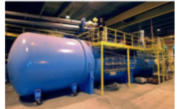
18 kW 4.5 K Refrigerator for LHC
