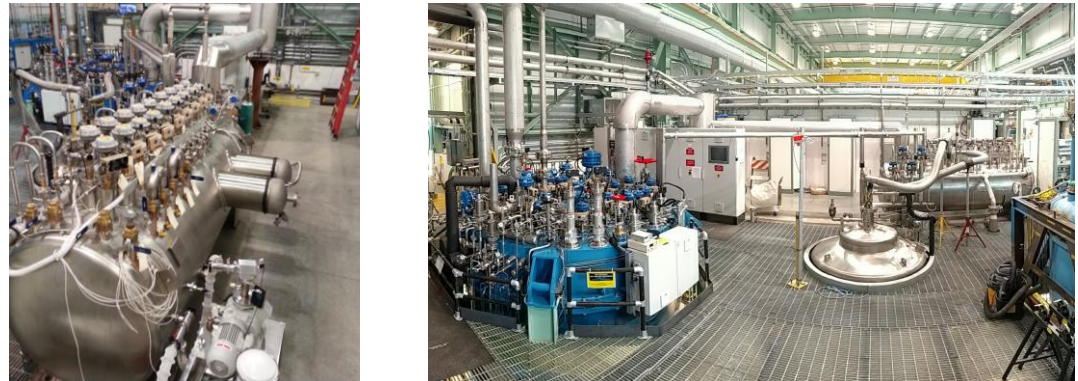
Figure 2: Pictures showing cryogenic distribution box, coldbox and Helium dewar at CMTF.
