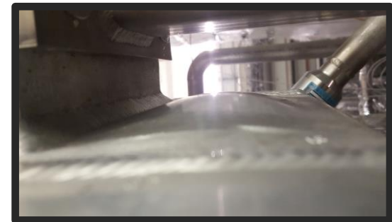
Figure 5: Picture of a damaged heat exchanger.
