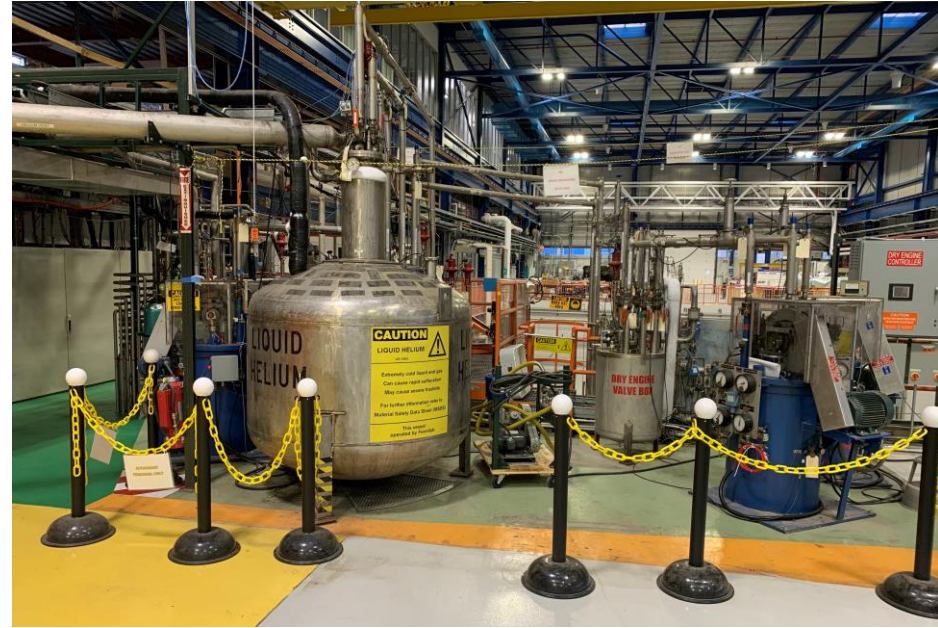
Existing cryoplant, with expansion engines, valve box and 2000-liter storage dewar
